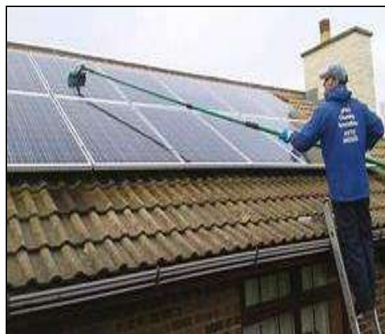
Fig 6: Manual Cleaning of PV panel.
